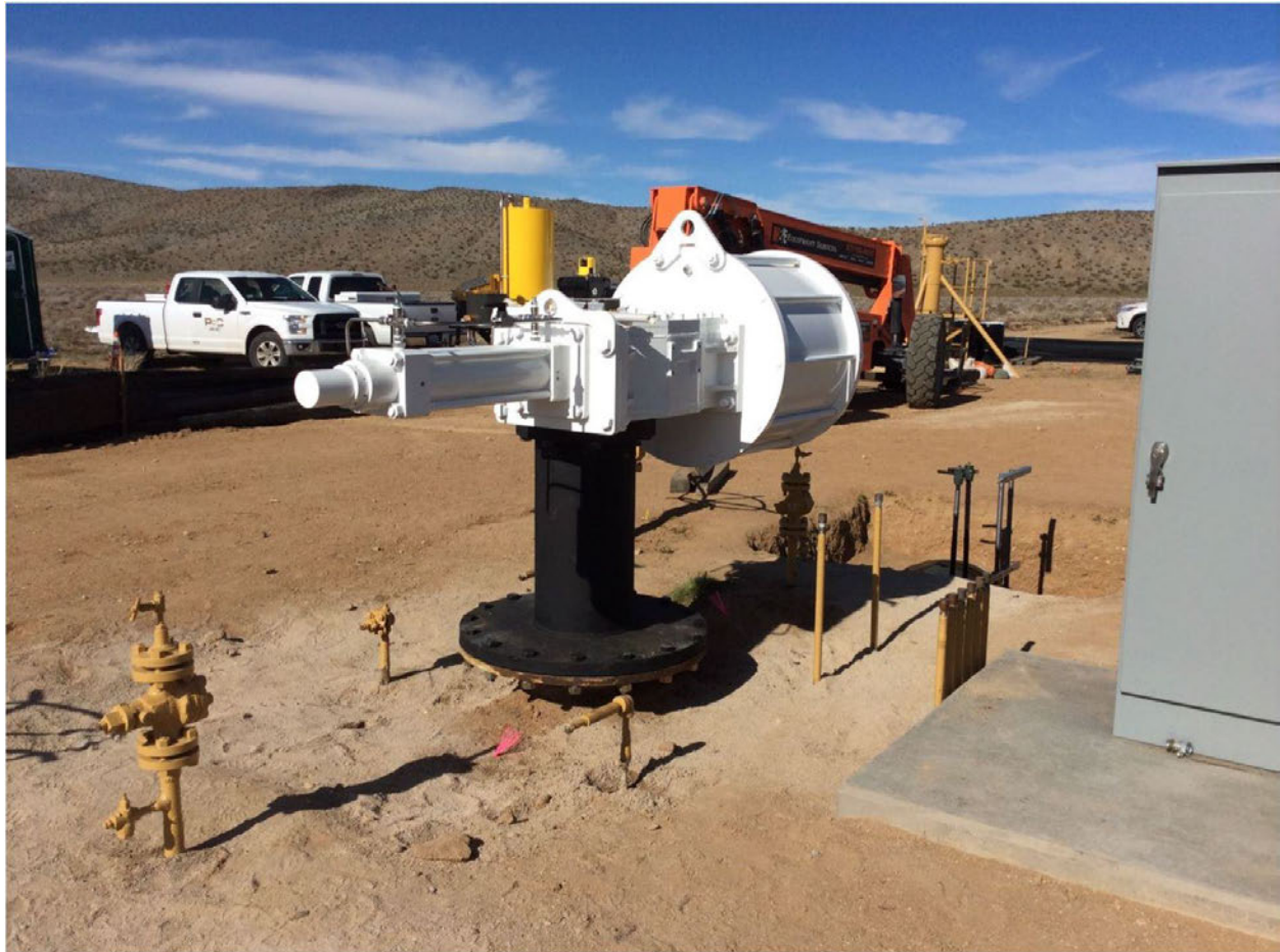
Figure 3: New Mainline Valve Actuator
