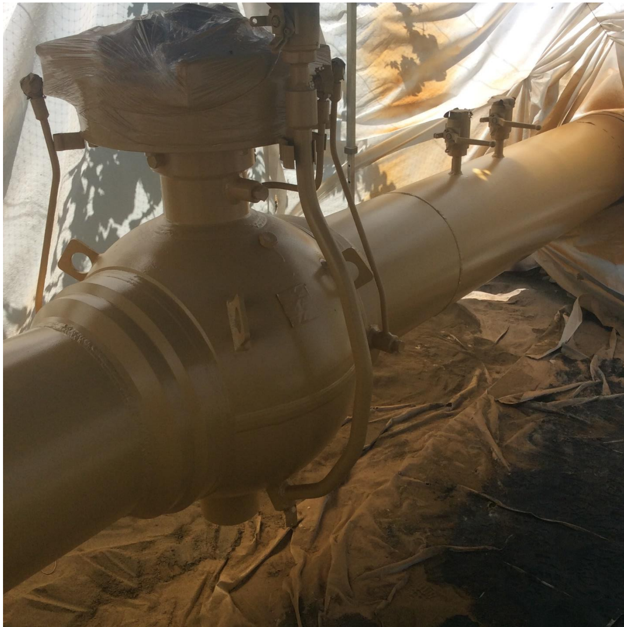
Figure 5: New Mainline Valve
