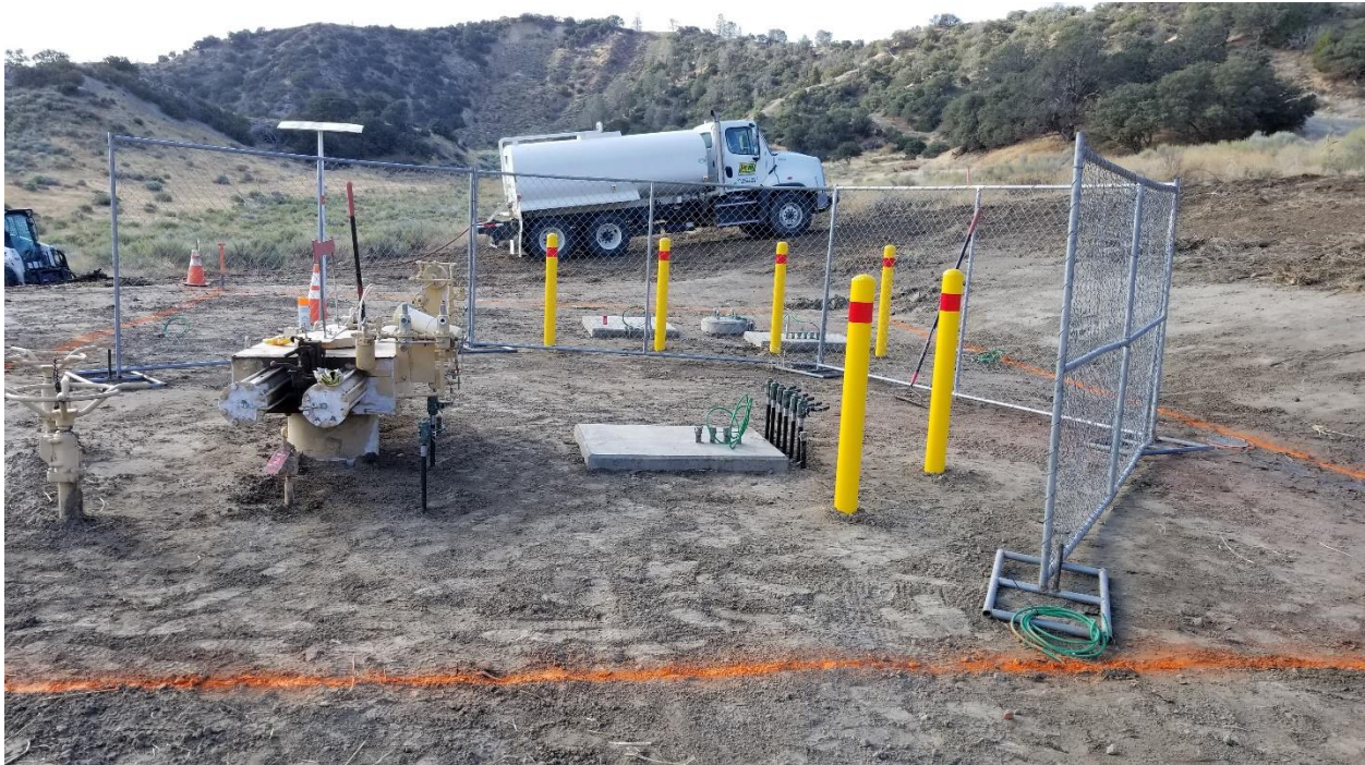
Figure 4: Project Site During Construction Foundation for the Linebreak Cabinet in the Foreground; Foundations for Solar Panel and Pole, New Battery Enclosure and New SCADA Enclosure in the Background
