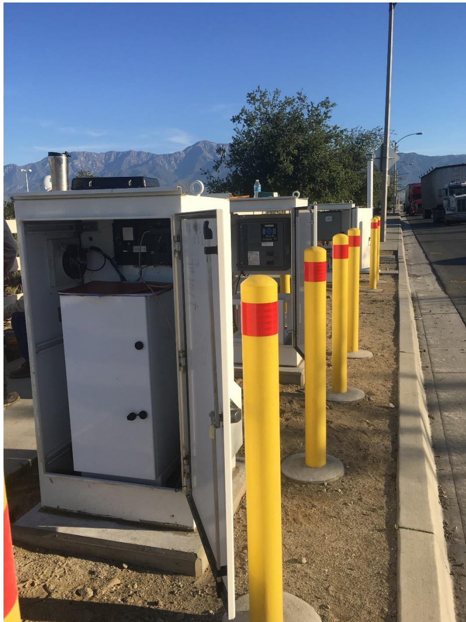
Figure 4: New SCADA Cabinet in the Foreground, New Battery Cabinet and Linebreak Cabinet in the Background
