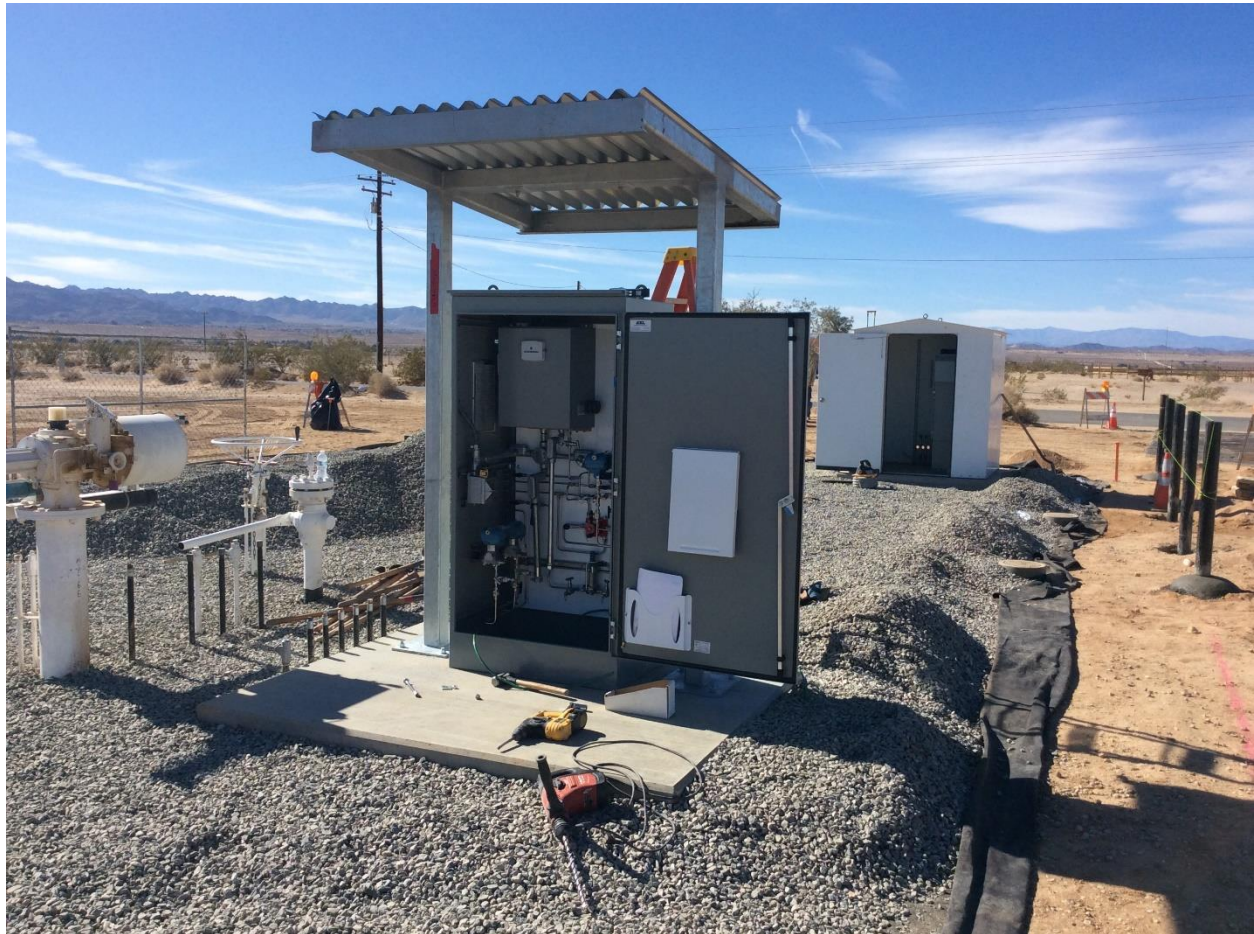
Figure 4: New Linebreak Cabinet in the Foreground, New Shelter in the Background
