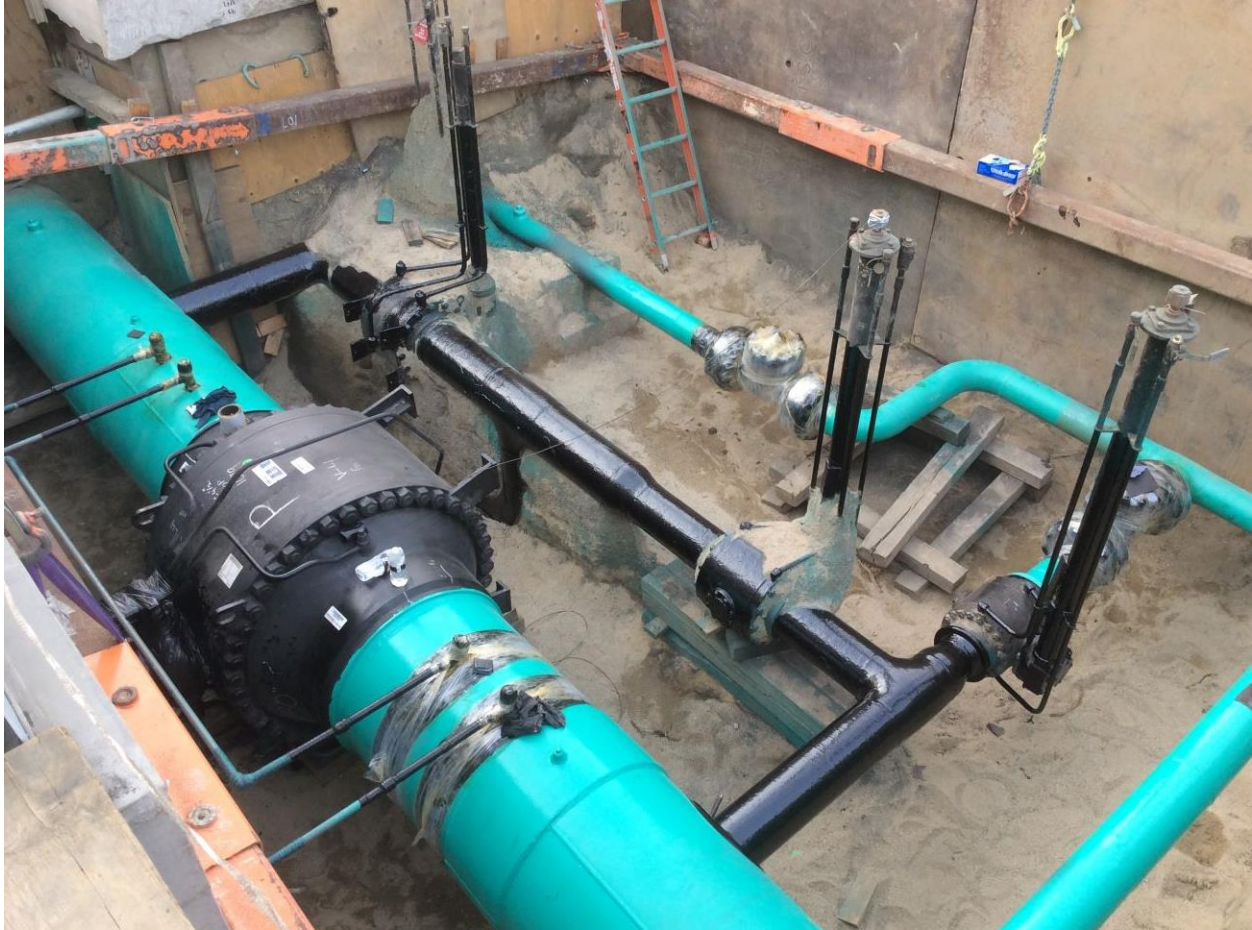
Figure 6: Faust Site: New Valves and Piping Assembly
