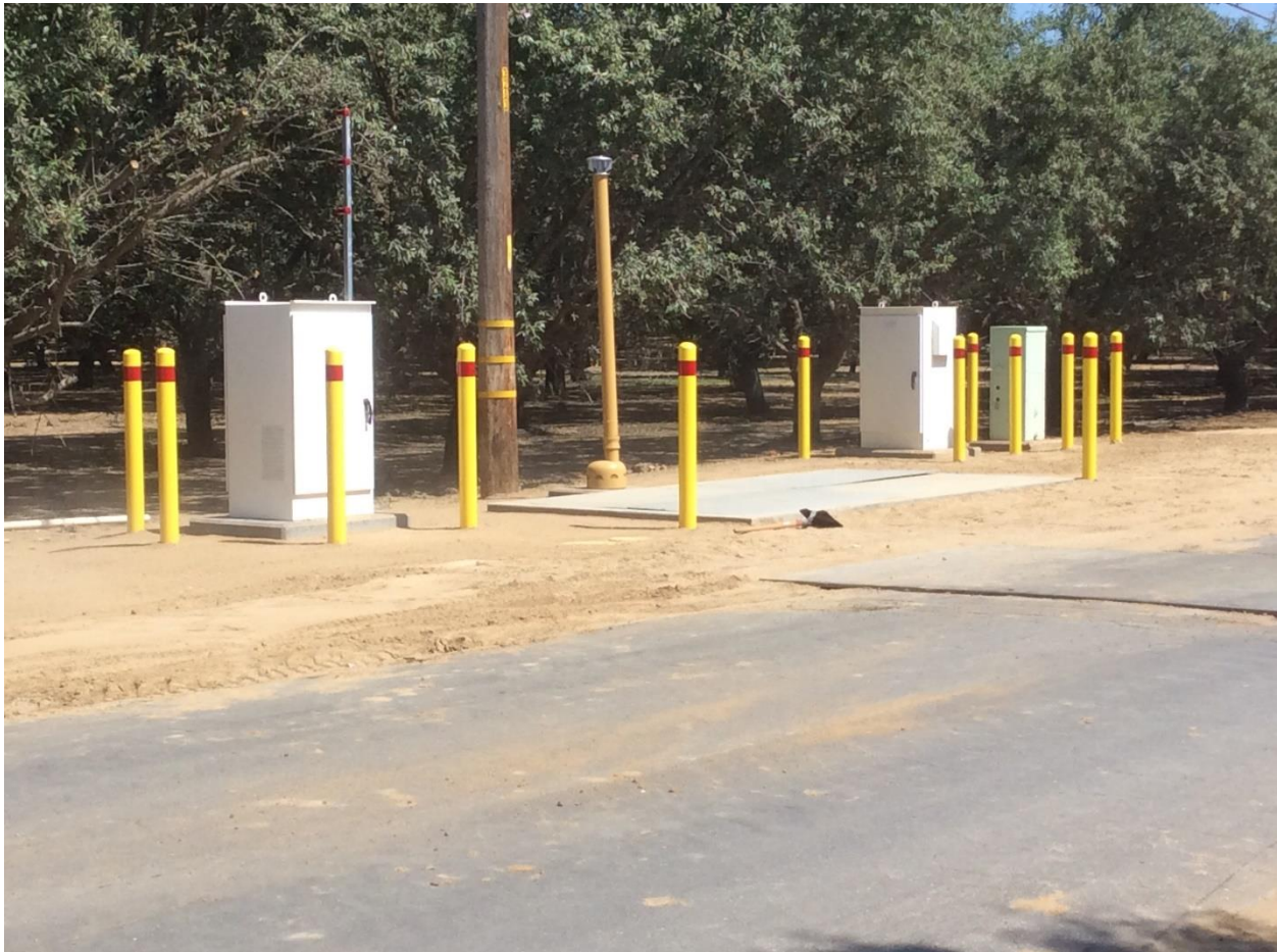
Figure 4: New Vault, Cabinets, and Bollards
