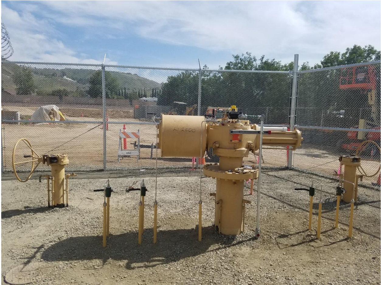
Figure 9: MLV 19 – Existing Actuator in New Fenced in Station
