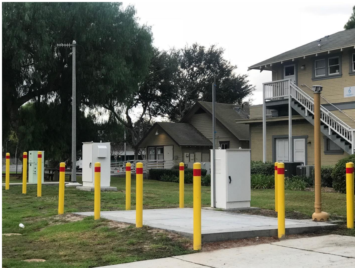
Figure 4: Project Site Post-Construction, New Vault in the Foreground, New Automation Equipment Cabinets in the Background
