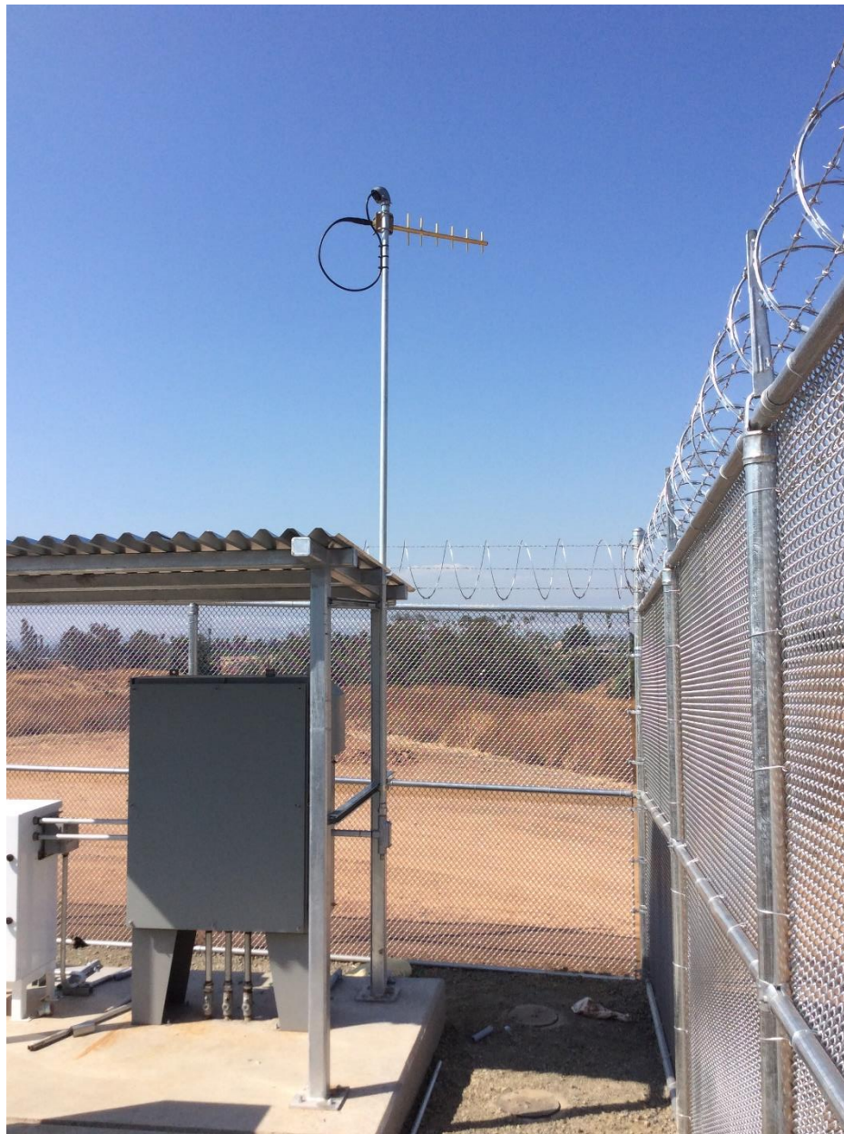
Figure 8: MLV 18 – New Linebreak Cabinet and Power Pole in New Fenced in Station
