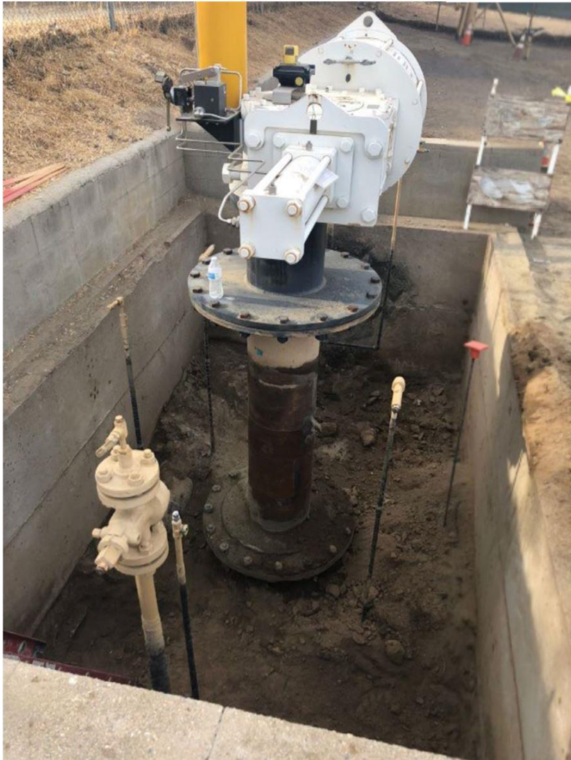
Figure 3: Existing Mainline Valve 4002-72.70-0 With Actuator
